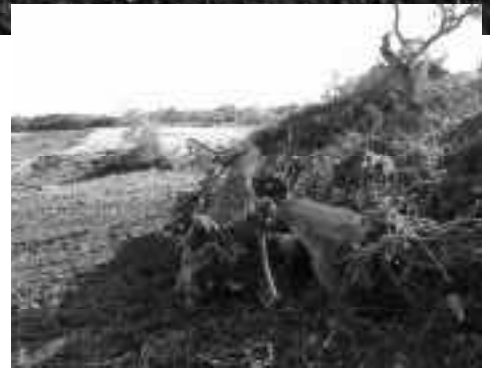
Scenes from Mopac: Large photo above: a grader has finished its job; Small photo above: some of the vegetation that has been removed to start drainage work.
